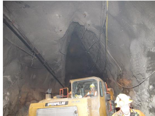
Discrete block failure
