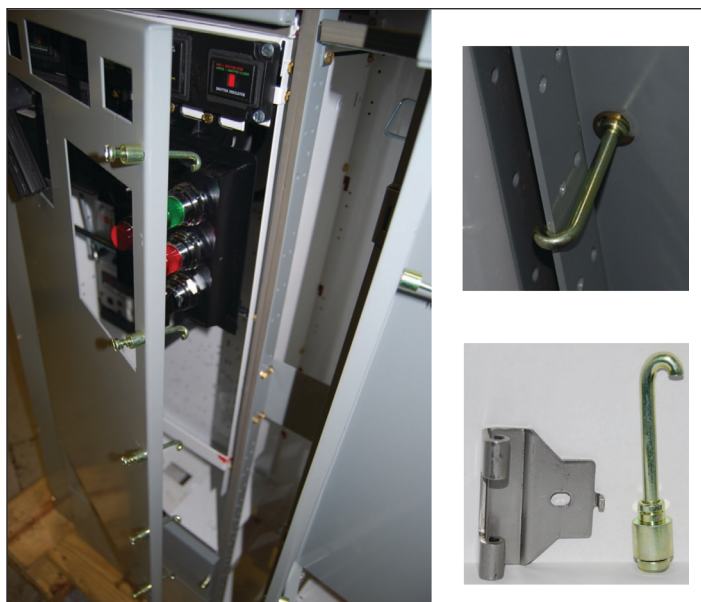
Figure 50. MCC unit and vertical wireway door latches and hinges
