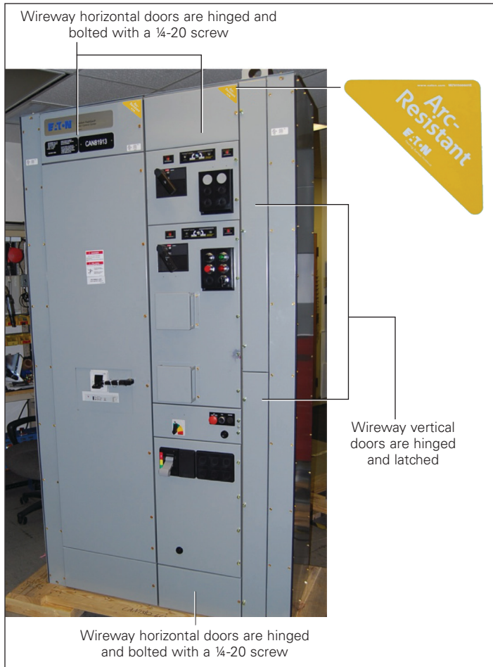
Figure 49. Arc resistant LV MCC—wireway doors and labeling
