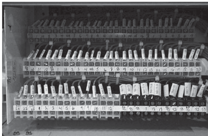
Figure 17. Master terminal block
