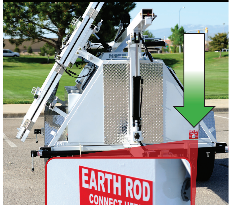
Figure 12: Grounding Rod Terminal on the left-front of unit
