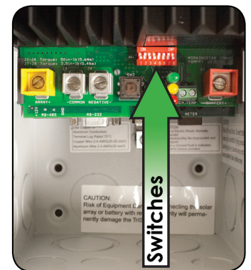
Morningstar Charger with Wiring Box Cover Removed.
