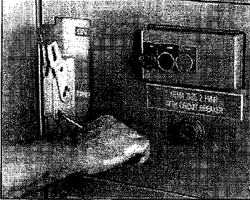
Figure 75: Operating Door Interlock Defeat Mechanism
