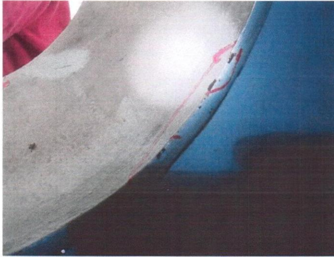
Internal Manway coating defects 2
