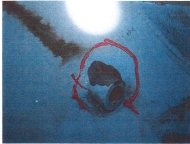
Coupling coating patch failure
