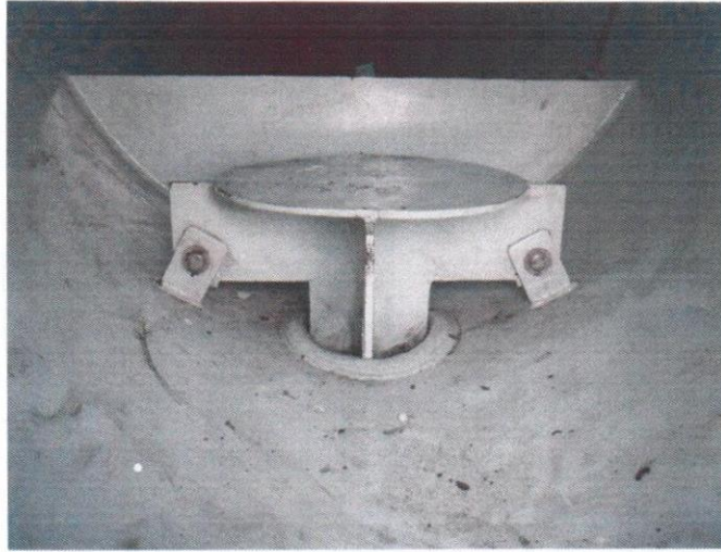
Vortex breaker on the outlet nozzle
