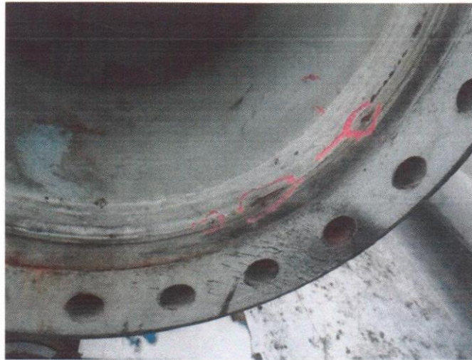
Manway Coating defects at the Gasket interface
