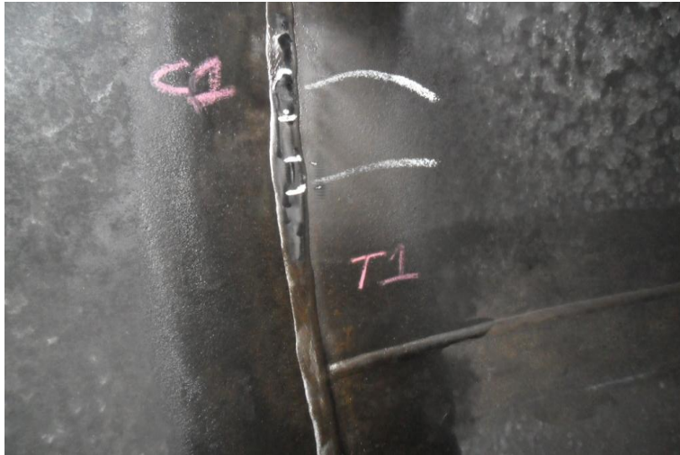
C1 / T1 Tee Weld Intersection Repair Weld in C2 Up 7" - 10" From T1
