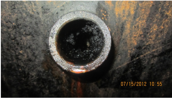
Photo 13: Buildup Inside Nozzles
