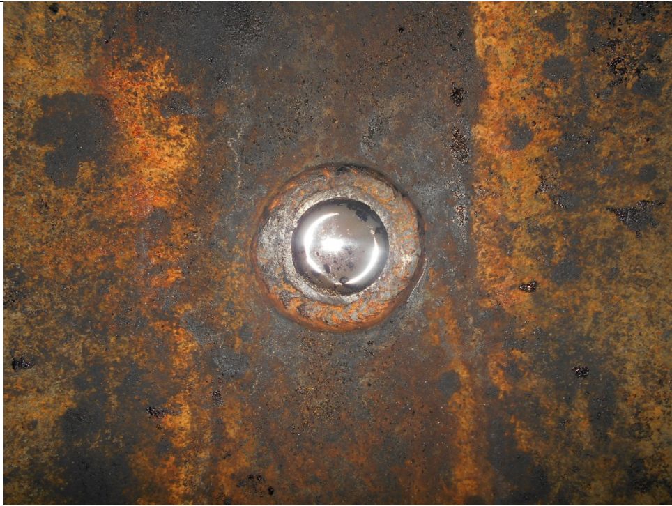
Figure 7 Lower Shell Drain Nozzle
