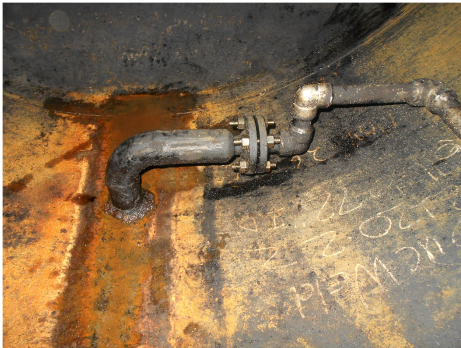
Figure 12 Glycol Heat Trace Nozzle and Piping
