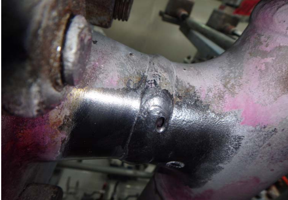
Leak Area: Weld Hole Thru
