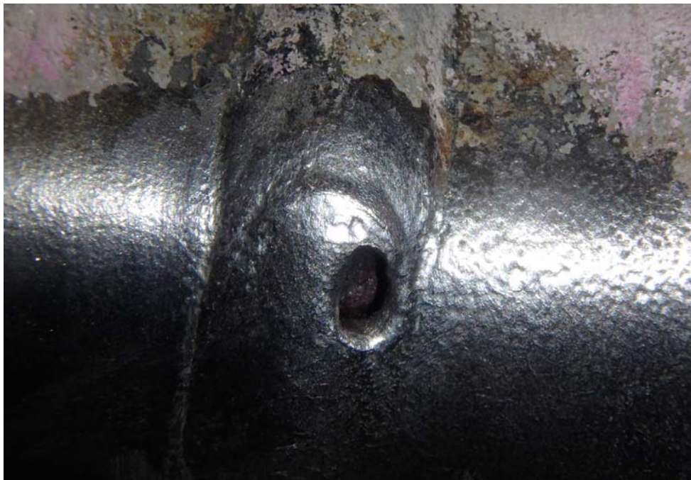
Leak Area: Weld Hole Thru (Macro)
