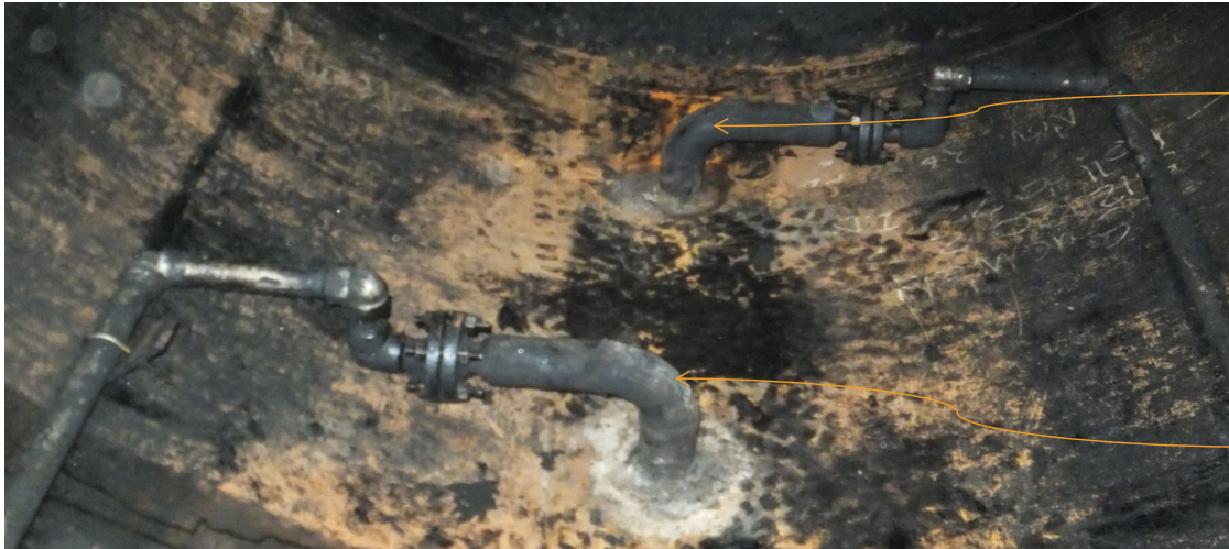
2" Inlet/Outlet Elbows (Carbon Steel) Schedule 160 Internal Min UT Thickness Found in mm
