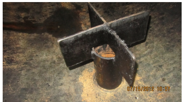
Photo 10: Vortex Breaker on Drain
