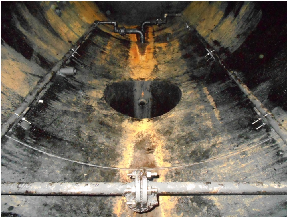
Figure 8 Glycol Heat Trace Lines and Boot
