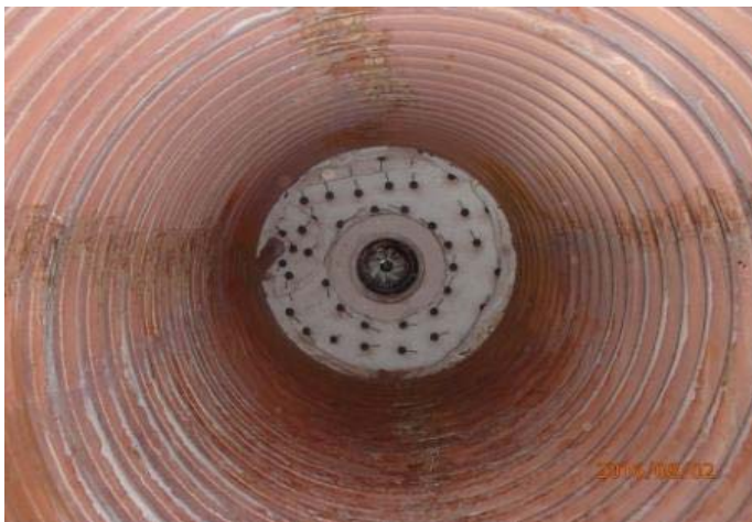
East Side Coil Overview
