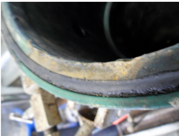
Photo 7: O-Ring Seal and Coating Chipped
