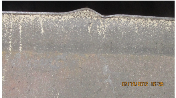
Photo 16: Mechanical Damage to Weir
