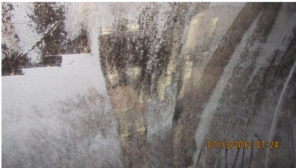
Photo 7: Heavy Buildup on Shell
