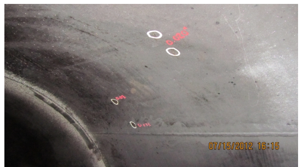
Photo 12: Corrosion Areas on Upper Shell
