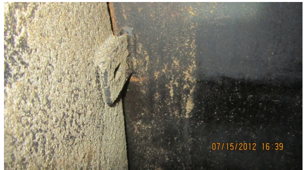
Photo 18: Saddle Missing Hardware
