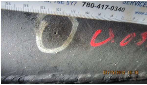
Photo 13: Corrosion on Upper Shell
