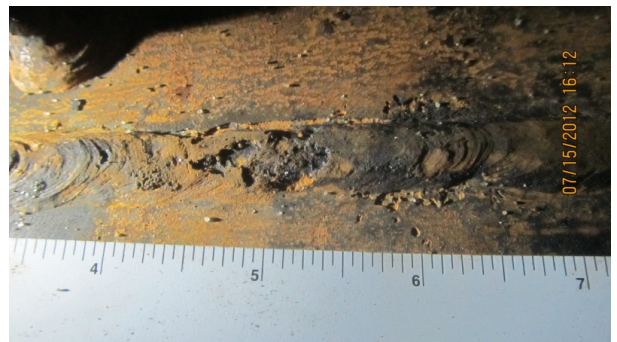
Photo 10: Corrosion on 0600 Position of Welds
