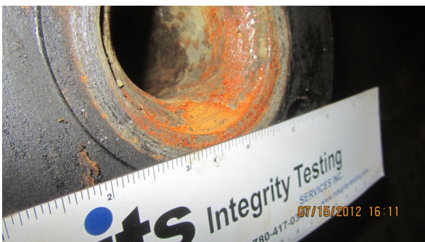
Photo 11: Corrosion on De-Sand Nozzle Internal
