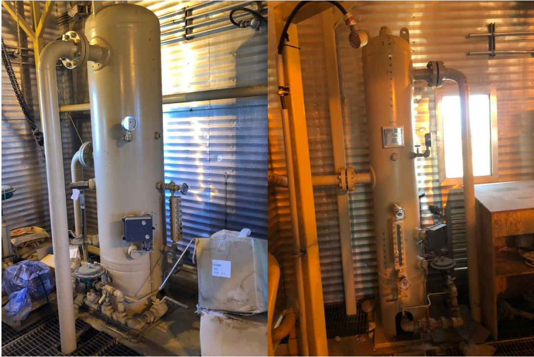
Stages 2 & 3 Suction Scrubbers
