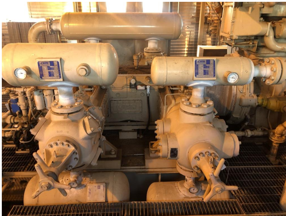
Waukesha Compressor showing Suction Bottle Stage 2&3
