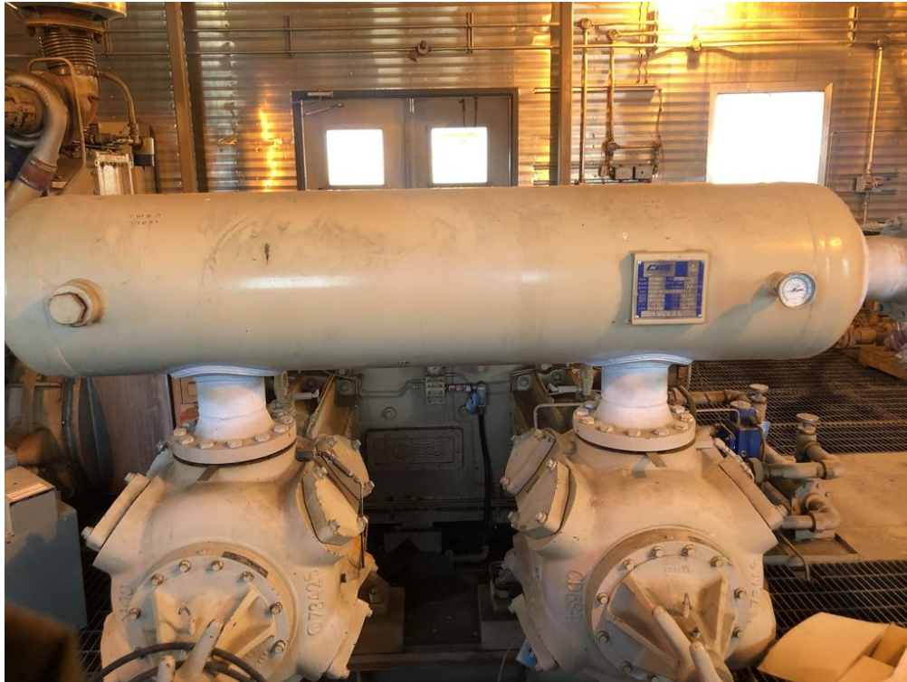
Waukesha Compressor showing Suction Bottle Stage 1
