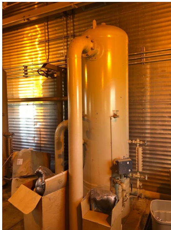
Stage 1 Suction Scrubber
