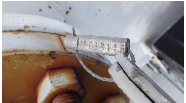
Photo 8 Description: PSV Valve Carsealed Open
