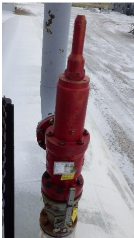
Photo 5 Description: PSV Overview
