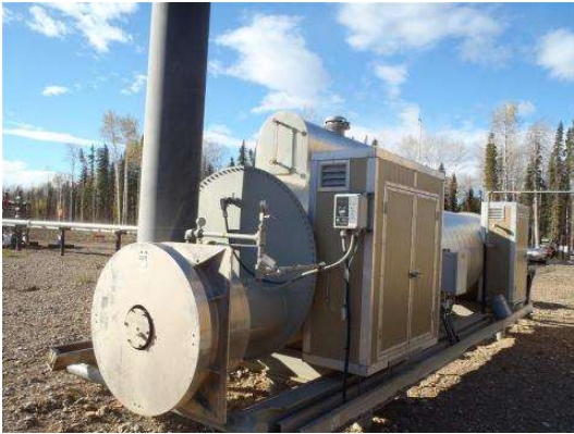
Line heater overview 1
