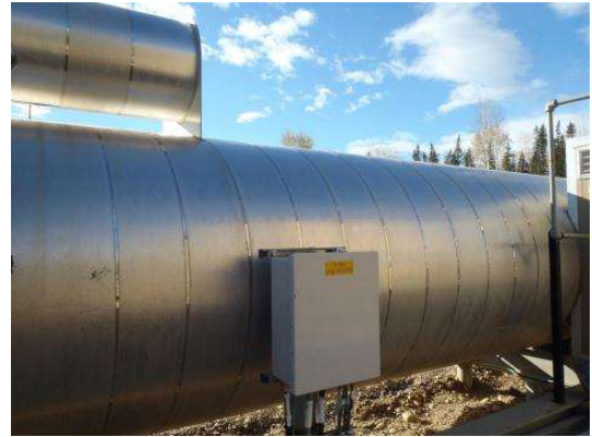
Line heater overview 2
