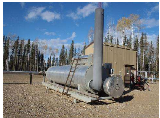
Line heater overview
