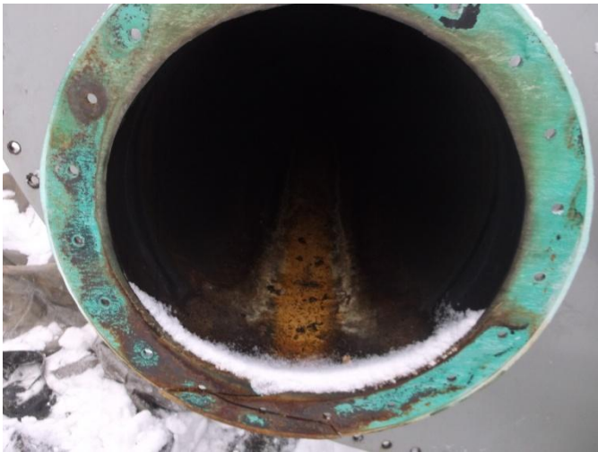
11 - H-500 LINEHEATER FIRETUBE BURNER SIDE DISCOLORATION
