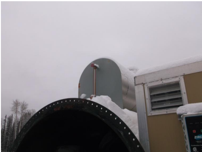
15 - H-500 LINEHEATER EXPANSION TANK & LEVEL GAUGE
