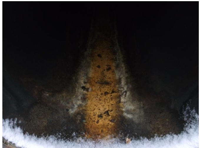
12 - H-500 LINEHEATER FIRETUBE BURNER SIDE DISCOLORATION
