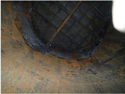
Bottom shell/demister overview
