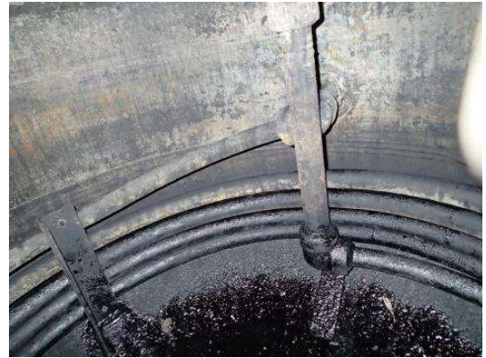
Bottom shell/head/glycol coil overview
