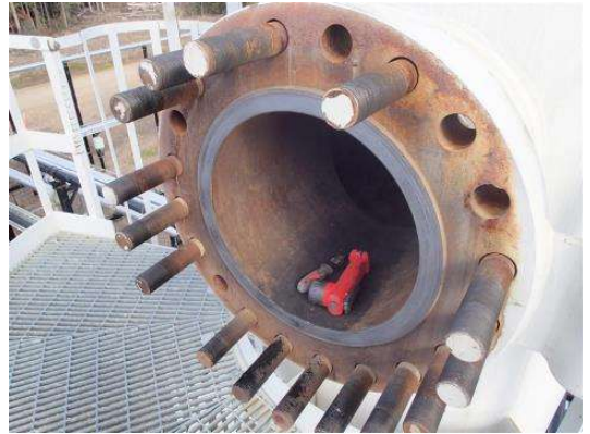
Top manway opening
