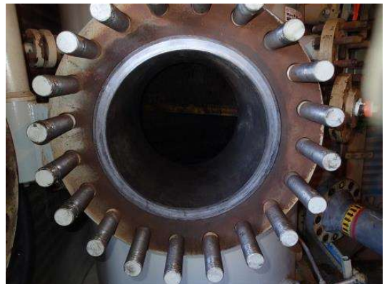
Bottom manway opening
