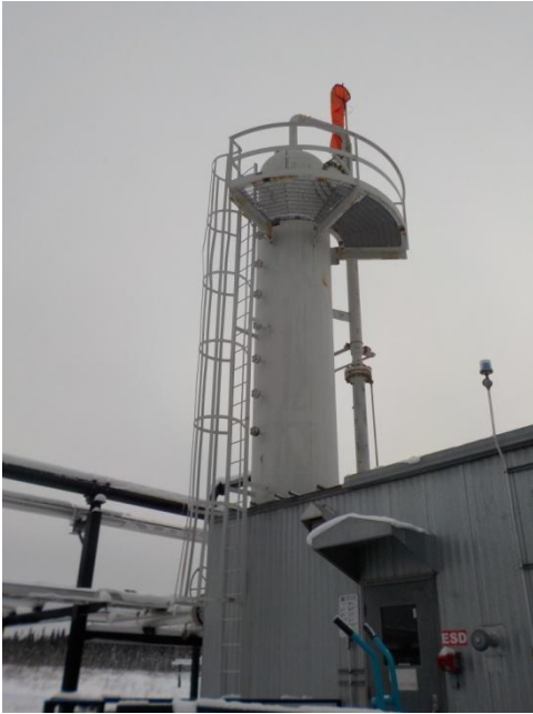
05 - T-500 GLYCOL CONTACTOR - OVERVIEW
