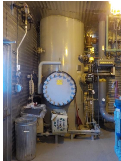
04 - T-500 GLYCOL CONTACTOR - OVERVIEW
