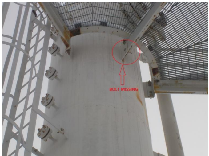
12 - T-500 GLYCOL CONTACTOR - ONE BOLT MISSING FROM PLATFORM BASE ATTACHMENTS
