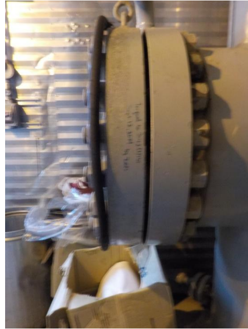
06 - T-500 GLYCOL CONTACTOR - MANWAY
