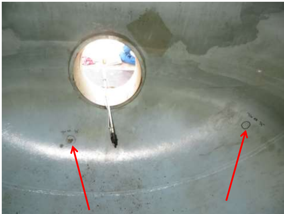
MANWAY HEAD AND 2 AREAS WITH COATING FAILURE
