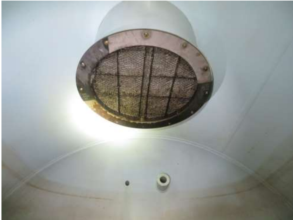
OUTLET, DEMISTER NOT REMOVED
