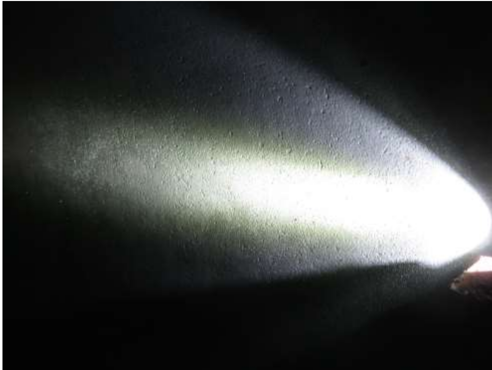
VIEW TYPICAL OF SMALL PITTING IN COATING AT 4:00 AND 8:00 THROUGHOUT SHELL
