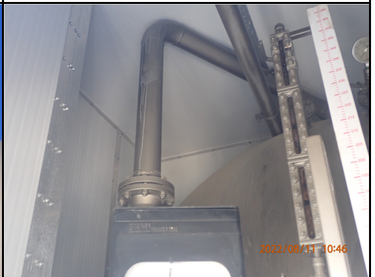
Gas Outlet Piping
