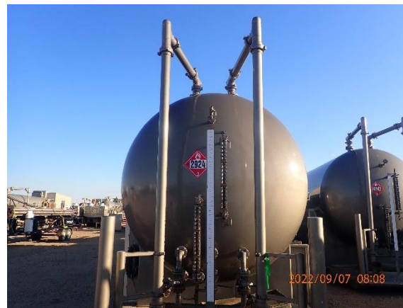
Overall view of Equipment
