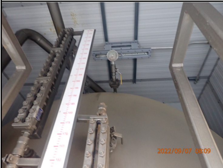
Gas Outlet Piping
