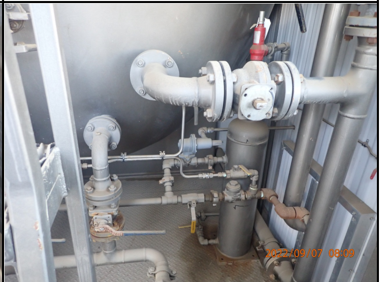
Liquid Outlet Piping
