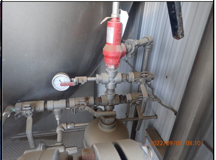
Gas Outlet Piping
