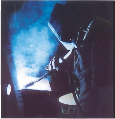
(46) ASME code welding stations providing Stick, MIG, TIG & sub-arc procedures
