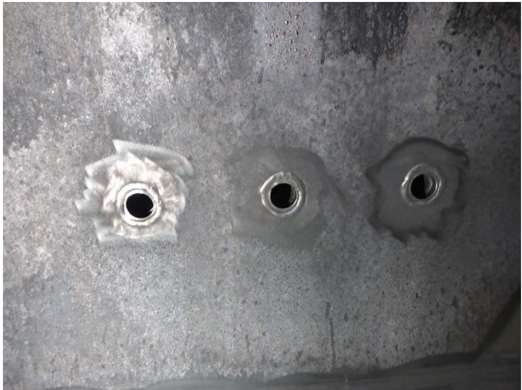
PSV Nozzles at 12 o'clock
