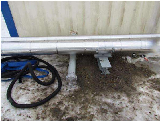
Piping from blow down vessel comes to a truck out point
