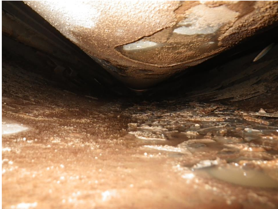
Bottom of furnace tube and shell (after cleaning)
