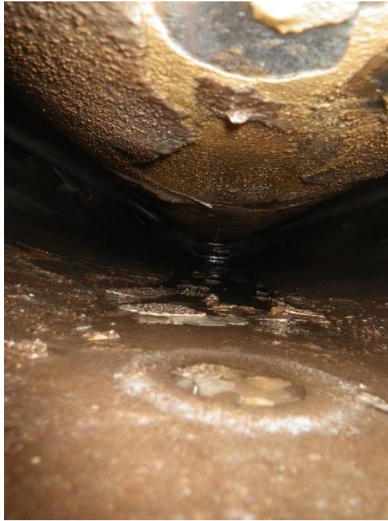
Bottom of furnace tube and shell (after cleaning)
