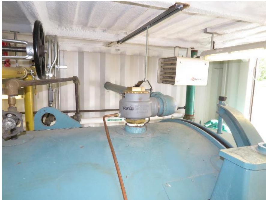
PSV and piping
