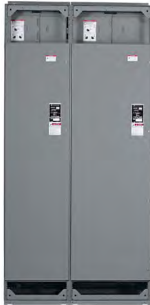
Figure 8B: Horizontal Wire Trough Covers Removed
