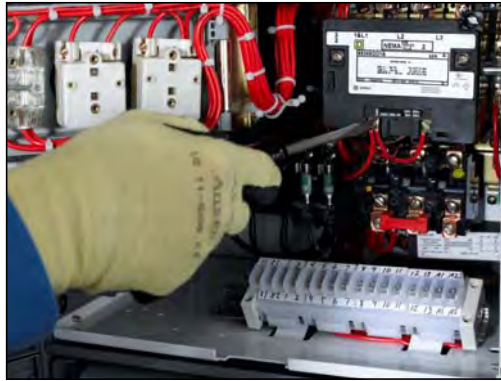
Figure 111 –Tightening Electrical Connections
