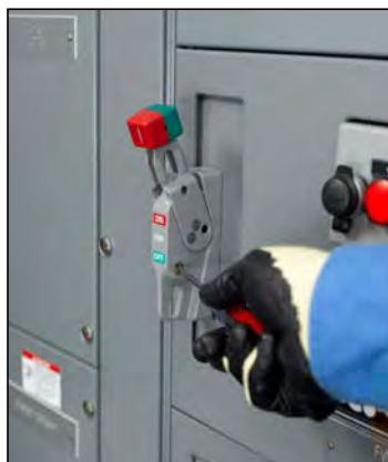
Figure 115 –Operating Door Interlock Defeat Mechanism
