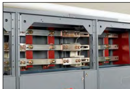
Figure 42 – Wireway Covers Removed and Horizontal Bus Barriers Open
