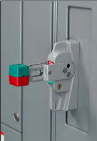
Figure 106 –Operator Mechanism in the Tripped Position
