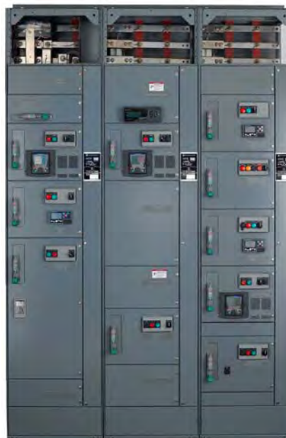
Figure 29 – Horizontal Wireway Covers and Bus Barriers Removed
