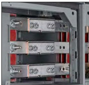
Figure 52 – Wireway Covers Removed and Horizontal Bus Barriers Open
