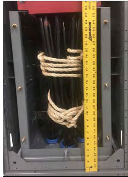
Figure 67 – Upper and Lower Cable Lacing Groups
