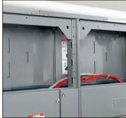
Figure 77 – Wiring in the Top Horizontal Wire Trough
