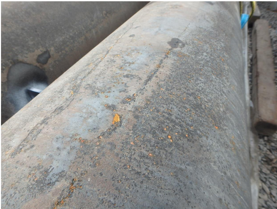
Figure 6: Pitting Present On Firetube
