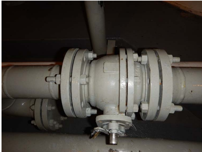
Missing Bolt on Flange
