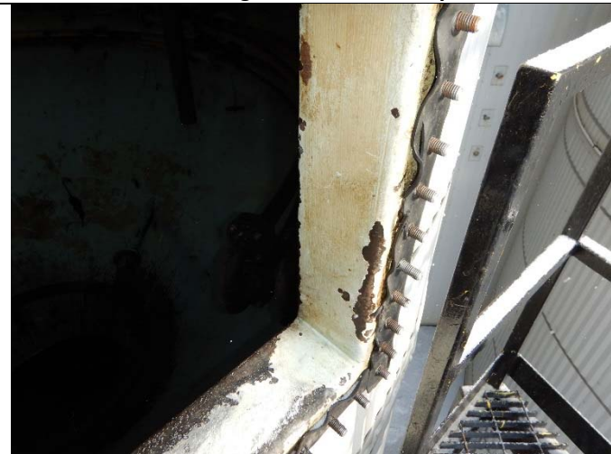
Coating Failure on Manway
