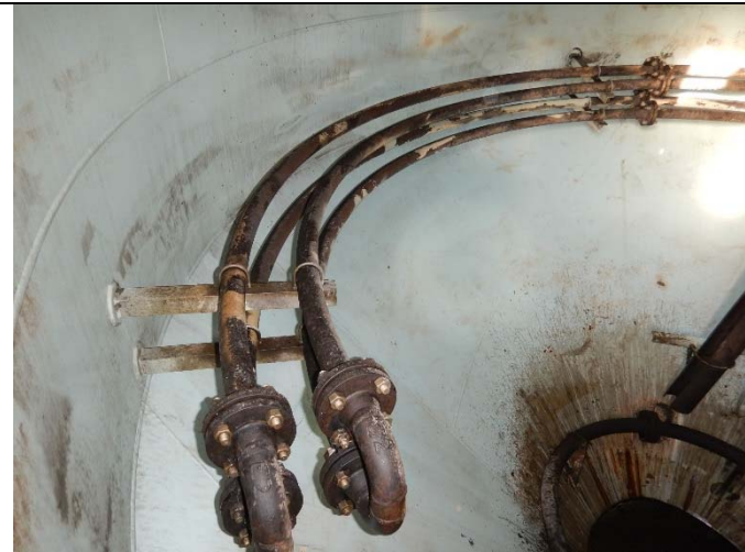
Internal Heating Coils
