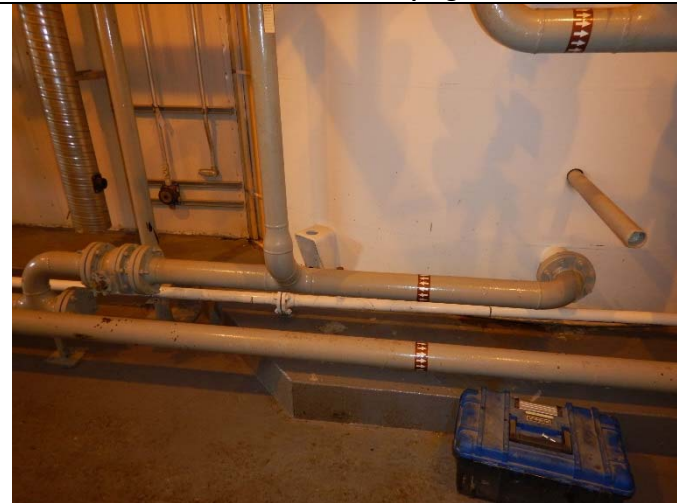
Missing Bolt on Flange
