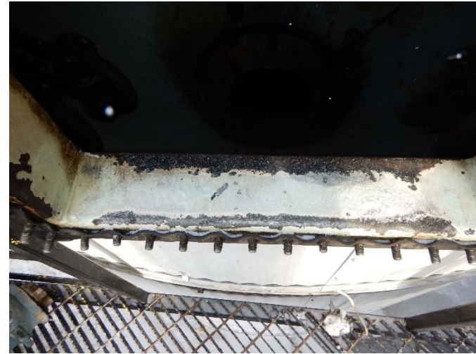
Coating Failure on Manway
