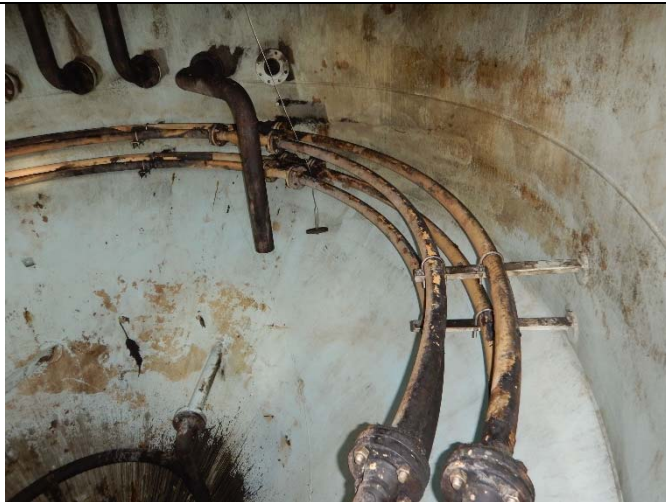
Internal Heating Coils
