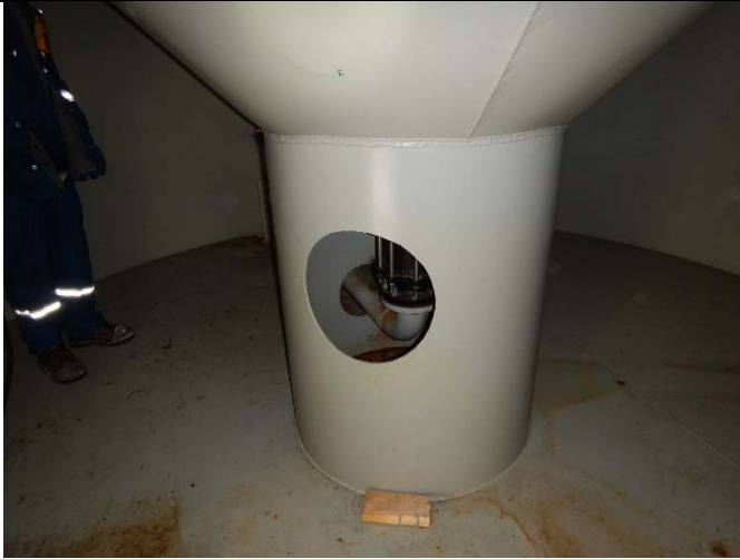
External Cone Bottom – Some Evidence of Prior Leaking
