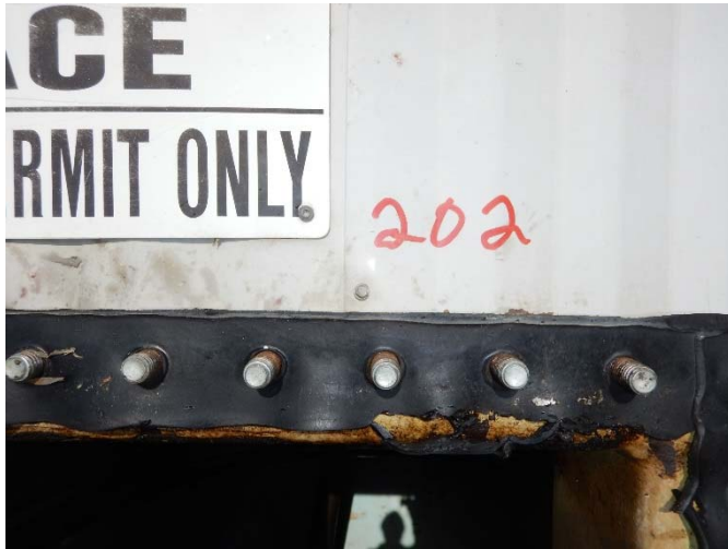
Coating Failure on Manway
