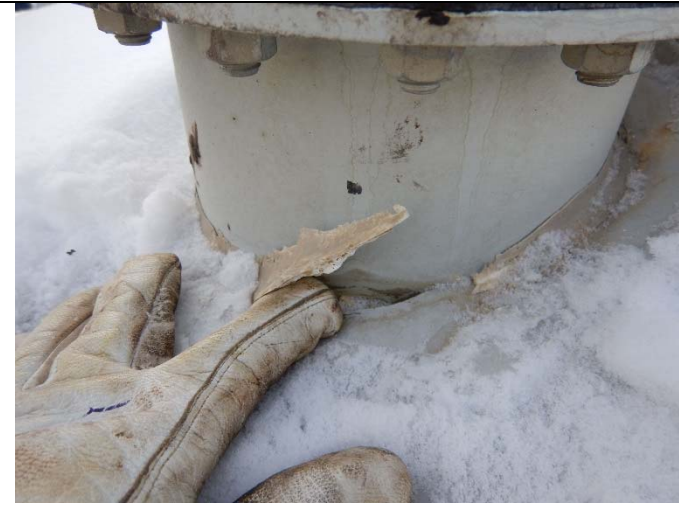
Deteriorating Seals on Cladding
