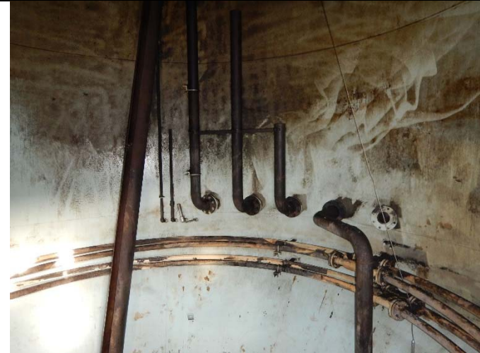
Tank Internal Piping
