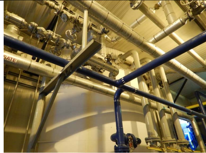
Tank External Piping
