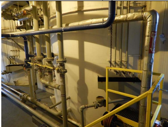
Tank External Piping
