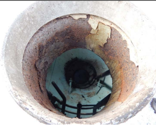
Coating Failure on ID of Thief Hatch
