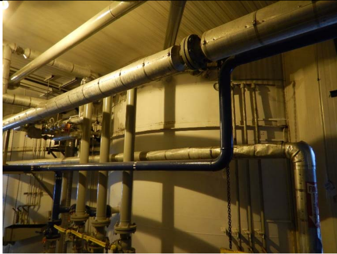
Tank External Piping
