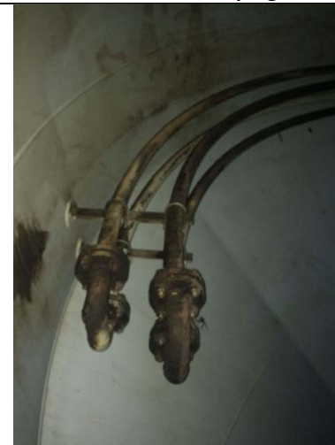
Tank Internal Steam Coils
