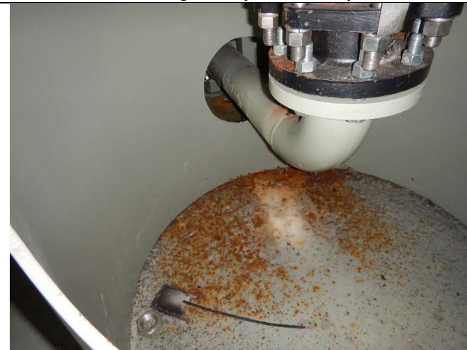
Evidence of Past Leakage of Bottom Cone
