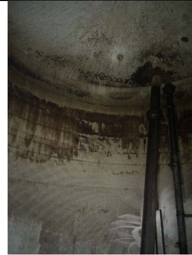
Tank Internal Piping
