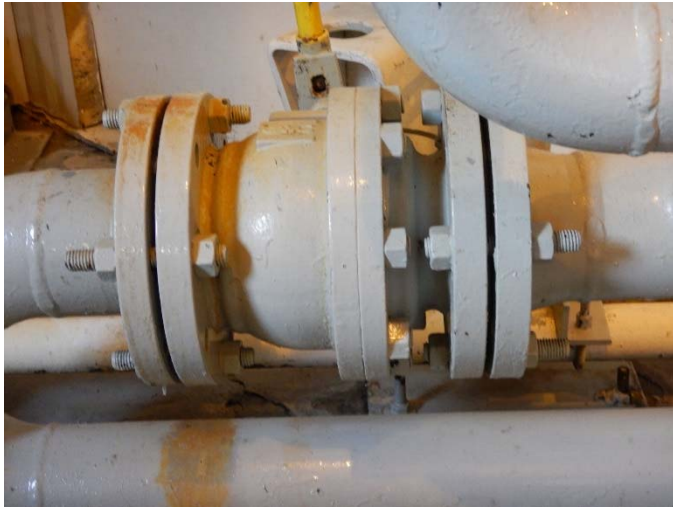
Cone Bottom Drain Valve Flange Missing Bolts
