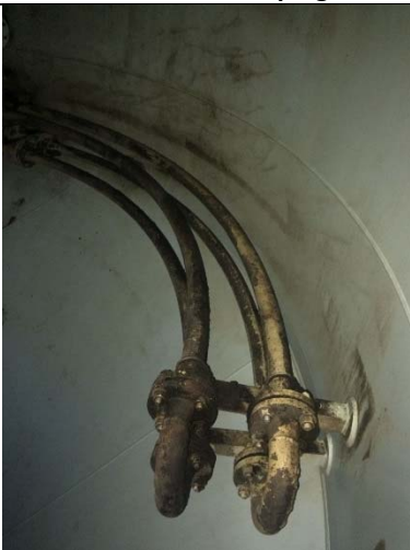
Tank Internal Steam Coils
