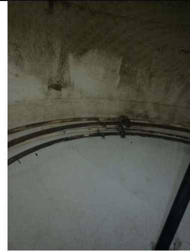
Tank Heat Coils
