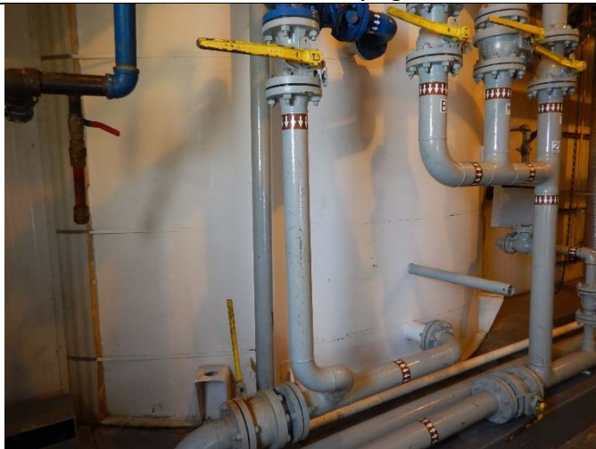
Tank External Piping
