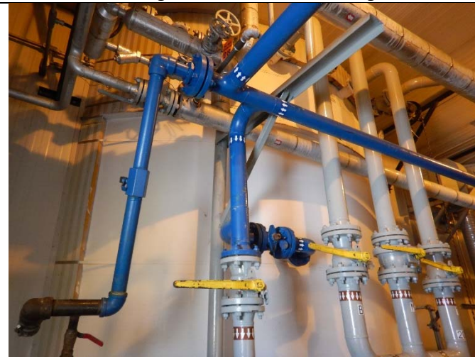
Tank External Piping
