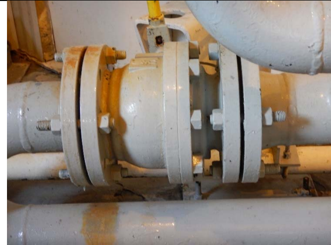
Missing Bolts on Drain Valve Flange
