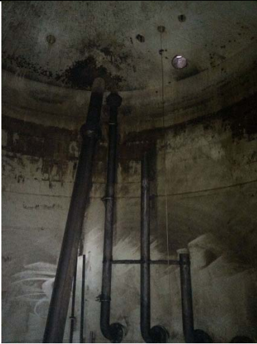
Tank Internal Piping
