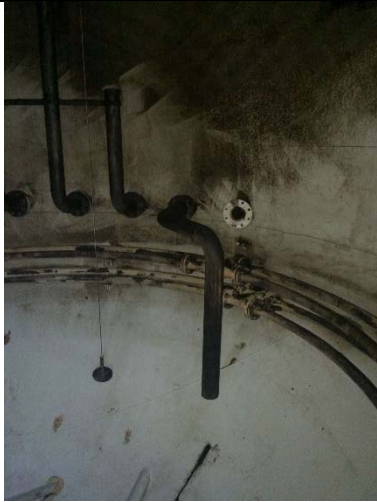
Tank Internal Piping
