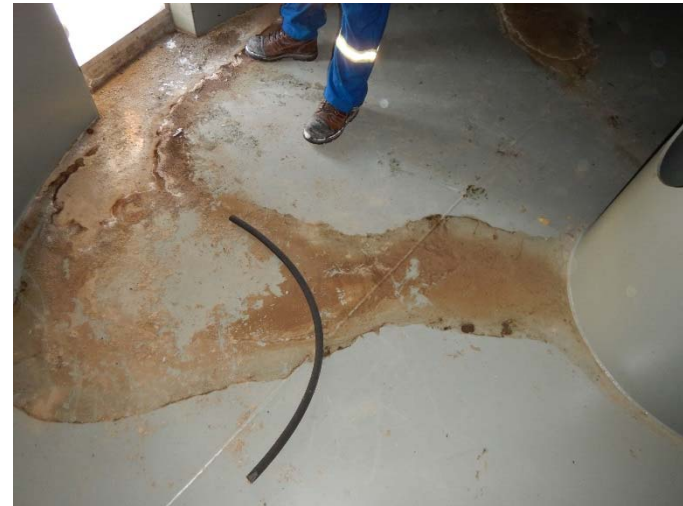
Evidence of Past Leakage
