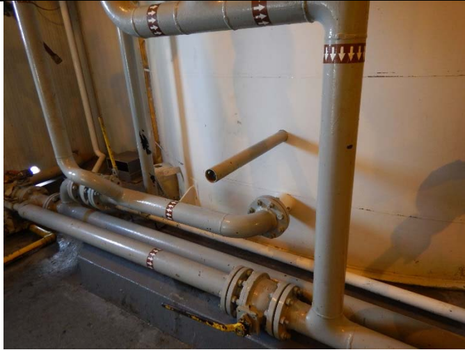
Tank External Piping
