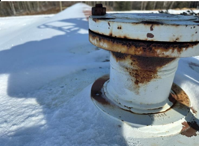
Photo 9: Flange surface corroded
