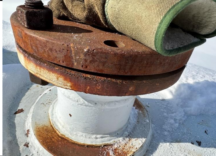
Photo 8: Untraceable blind flange to be removed/replaced
