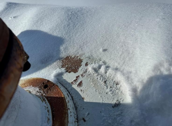
Photo 7: Corrosion around weepholes
