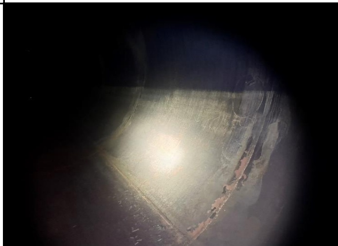
Photo 12: Debris in vessel
