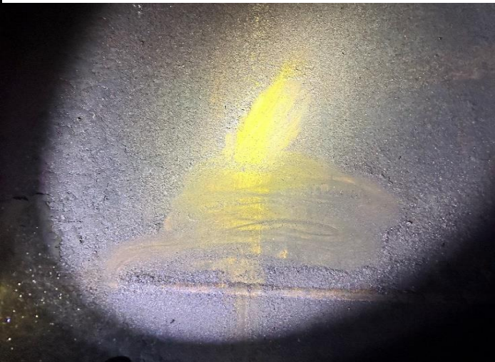
Photo 9: Debris in vessel
