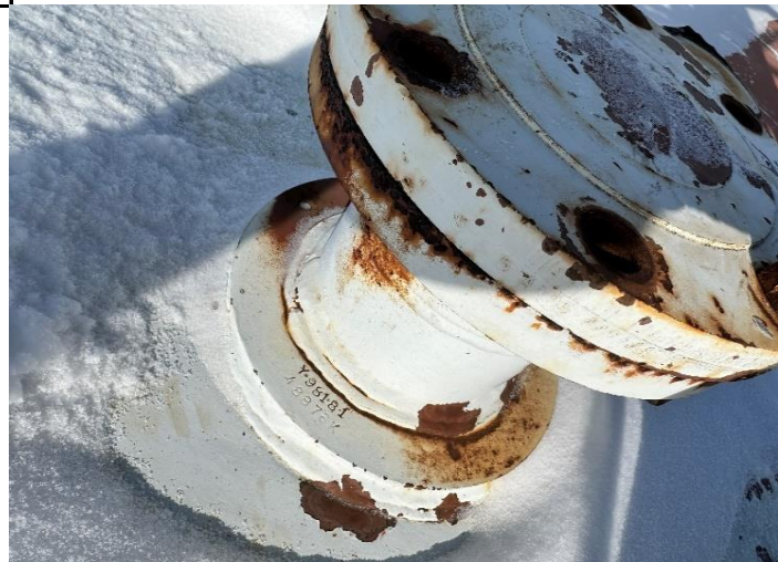
Photo 10: Blind flange installed upside down
