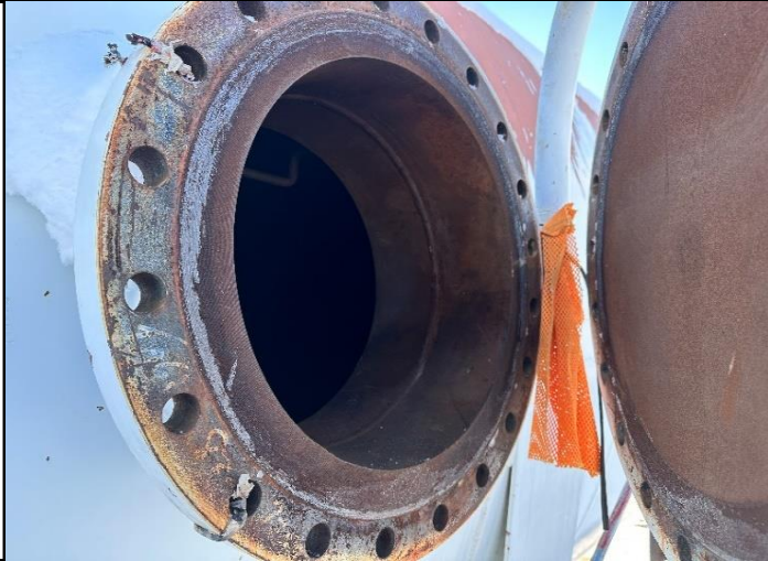
Photo 2: Manway gasket face
