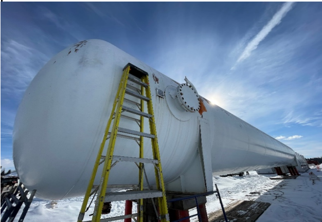
Photo 9: Manway measured WT at bottom on 20" pipe
