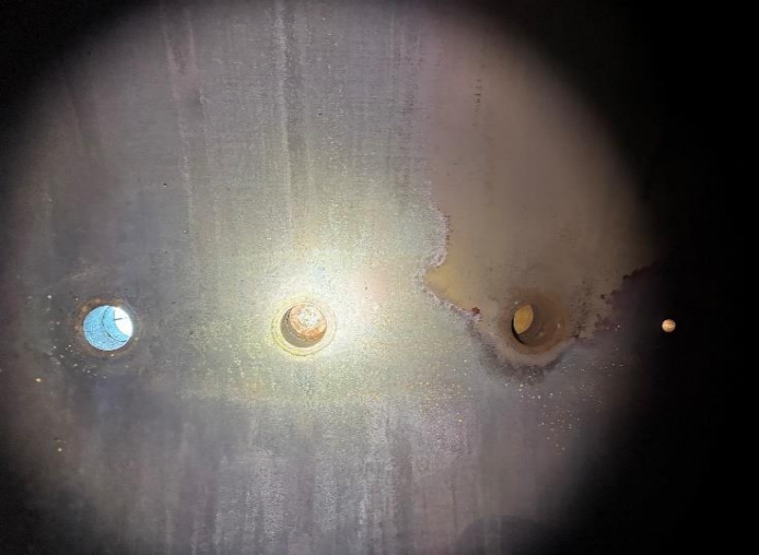
Photo 7: PSV nozzles on top of vessel in good condition
