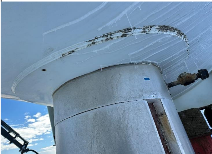
Photo 5: Insulated sump, repad
