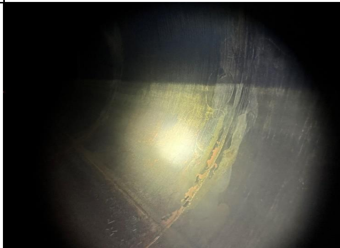
Photo 10: Debris in vessel
