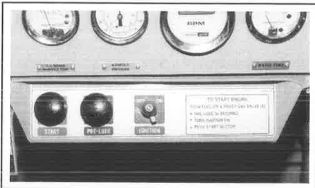
Figure 2.50-10. 16 Cylinder Control Panel
