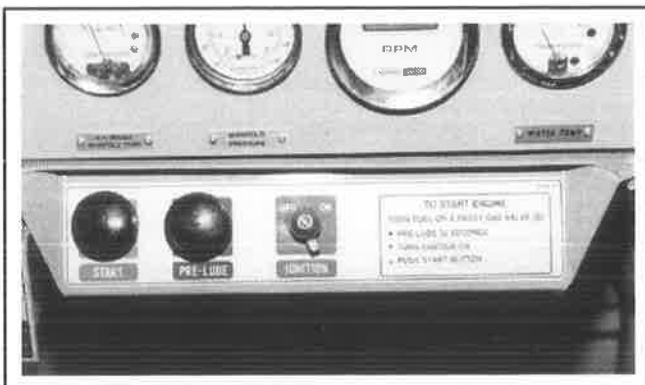
Figure 2.50-10. 16 Cylinder Control Panel
