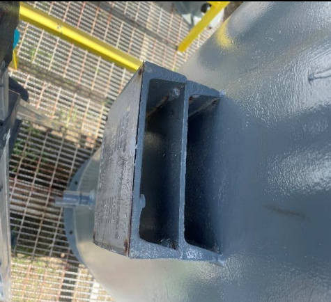
Photo 9: Nameplate has 2 mounts
