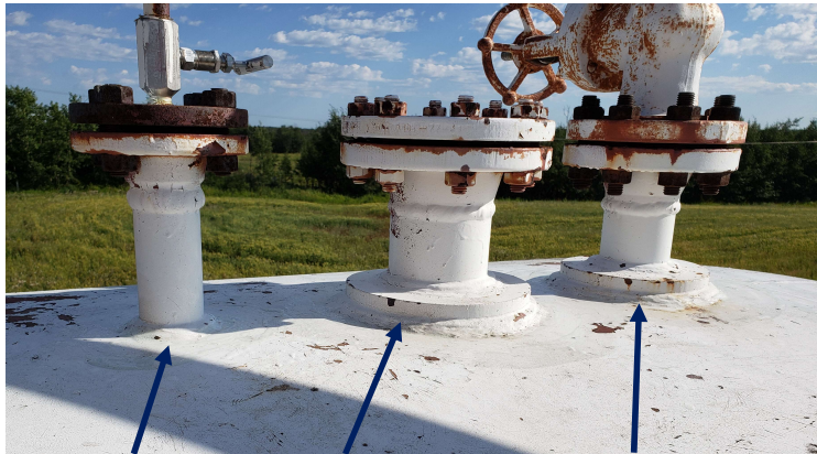
UT 10 2" Nozzel UT 11 4" Nozzel with Repad No Inspection UT 12 3" Nozzel with Repad No Inspection
