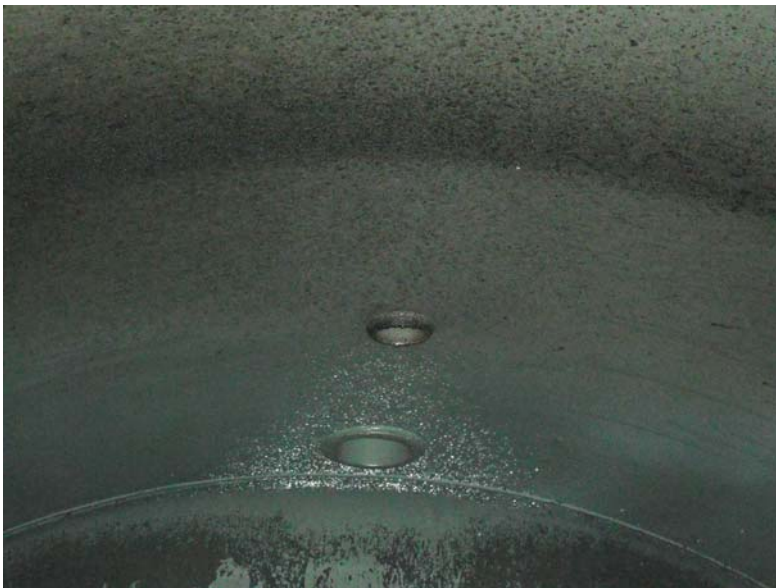
Grand Forks-FWKO_ Internal Nozzles
