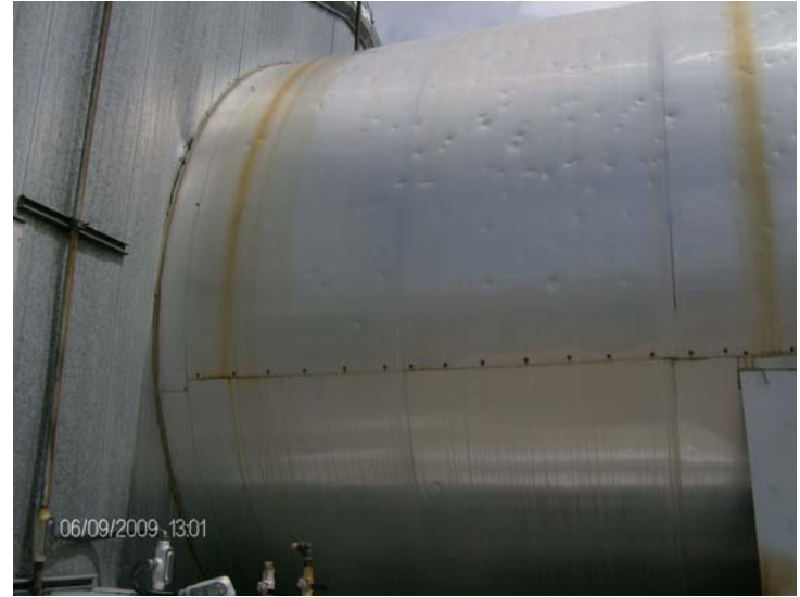
Grand Forks-FWKO_ Dimpled Insulation
