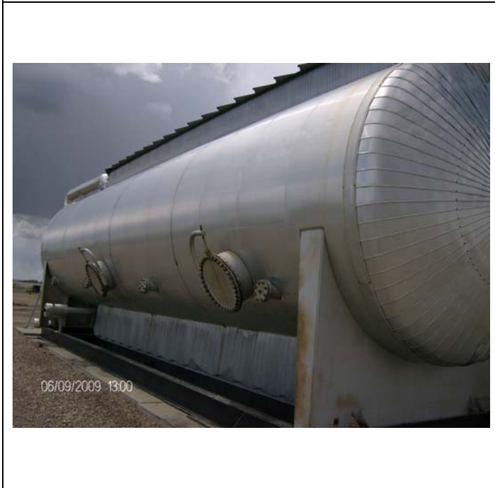
Grand Forks-FWKO_Outside Bldg.
