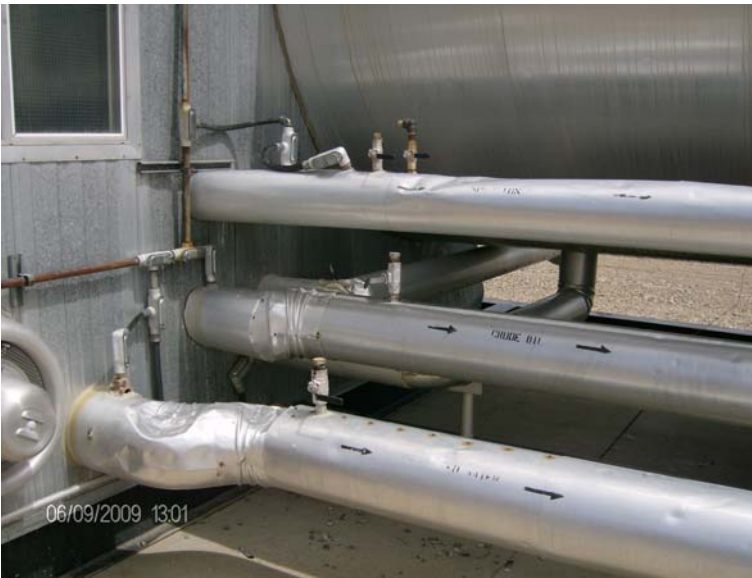
Grand Forks-FWKO_ Crushed Piping Cladding
