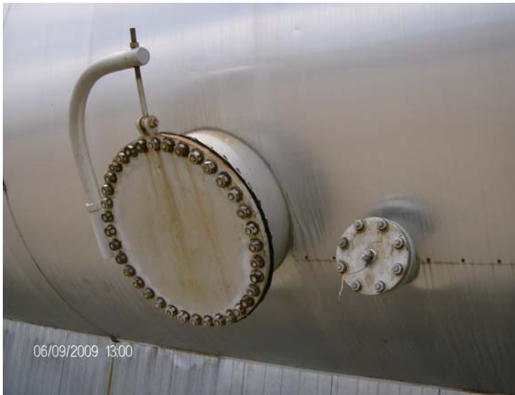
Grand Forks-FWKO_Broken Anode Wire
