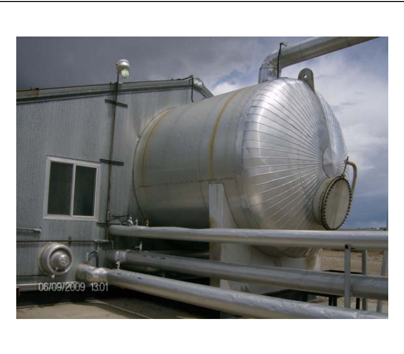
Grand Forks-FWKO_Outside Bldg.
