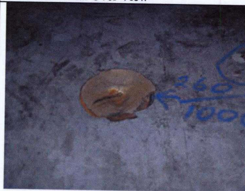
Lower Shell 260/1000 pitting
