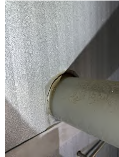
Insulation Not Sealed at Nozzle/Building Interface
