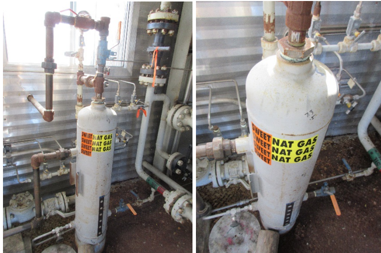
Support and Paint Condition
