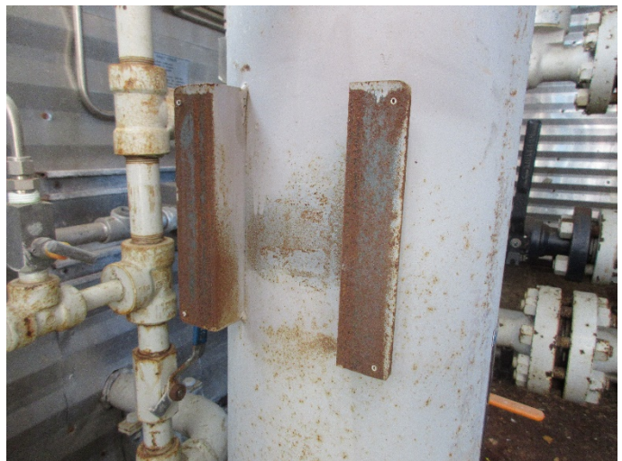
Missing Data Plate
