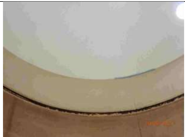
Rare-ST82252-AST-PrePurchase-Int-Past Coating Repairs1-Typical-10-06-2021.JPG
