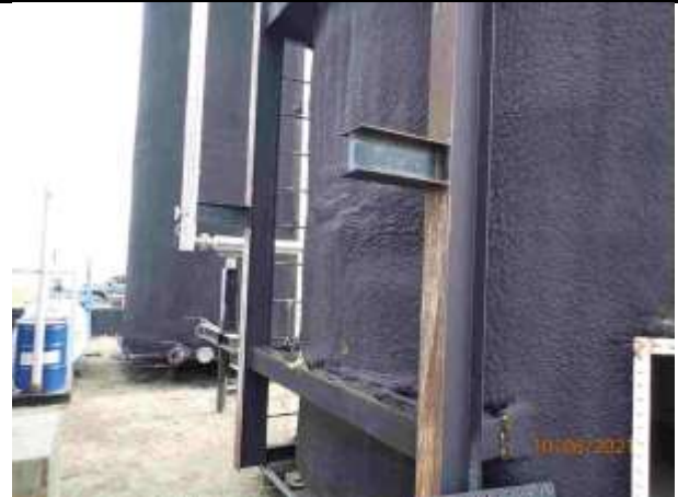
Rare-ST82252-AST-PrePurchase-Ext-Piping Supports on Transportation Skid-10-06-2021.JPG
