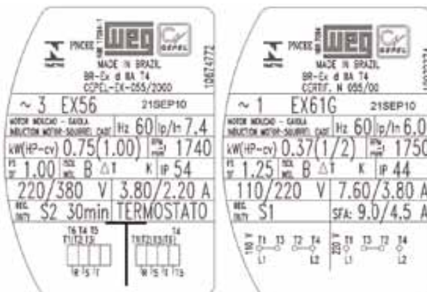
Figure 2.3 - Nameplate of fuel pump motor.
