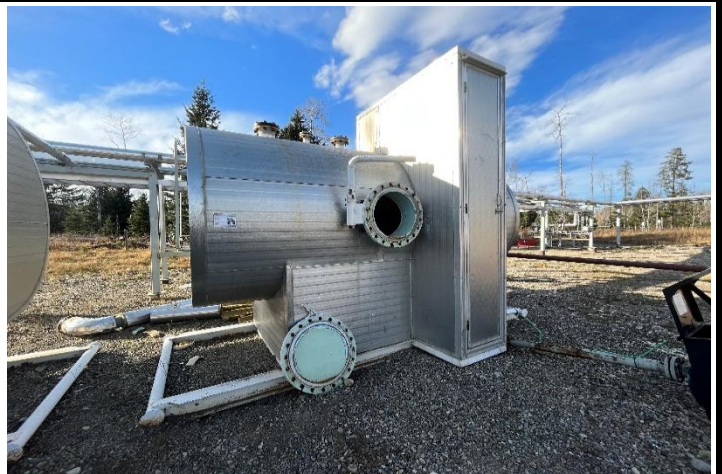
General over view of insulation & skid.
