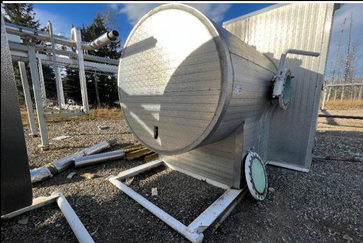
General over view of insulation & skid.
