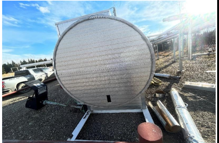
General over view of insulation & skid. (Light hail dents on head)
