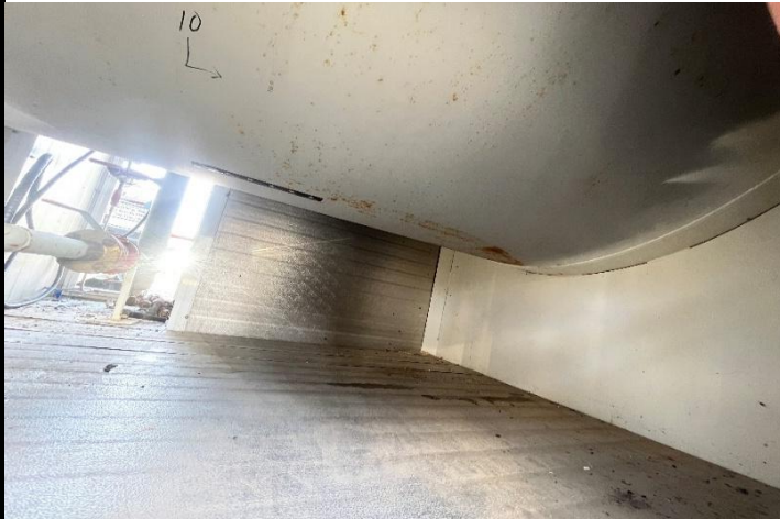
External shell belly view in crawl space. (Superficial rust specs)
