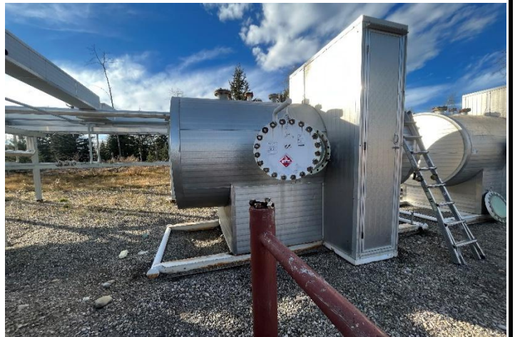
General over view of insulation & skid.
