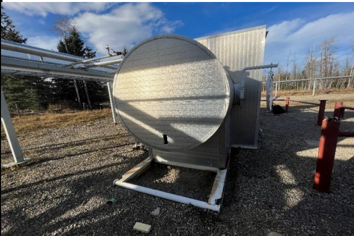
General over view of insulation & skid.
