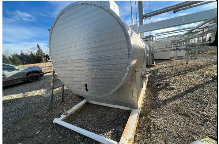
General over view of insulation & skid. (Light hail dents on head)
