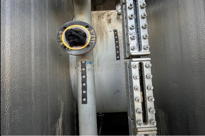
External mid/upper shell view from cabinet.
