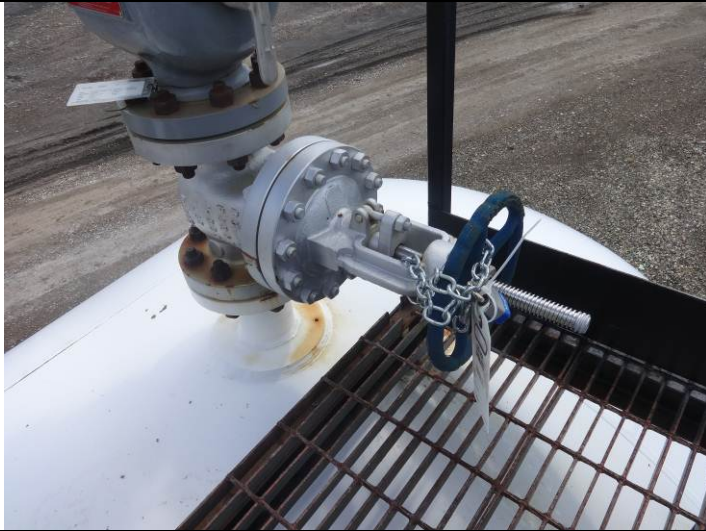
PSV Block Valve, locked open
