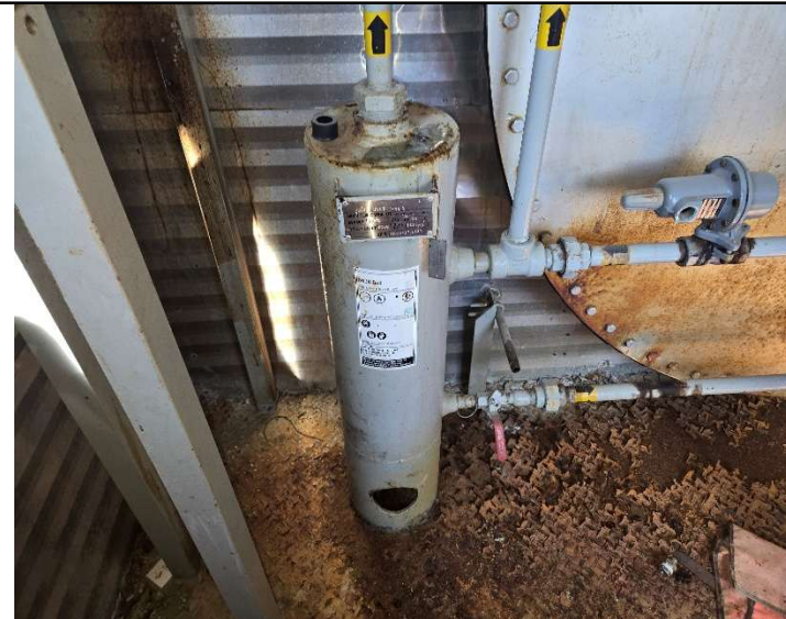
Fuel Gas Scrubber Overview
