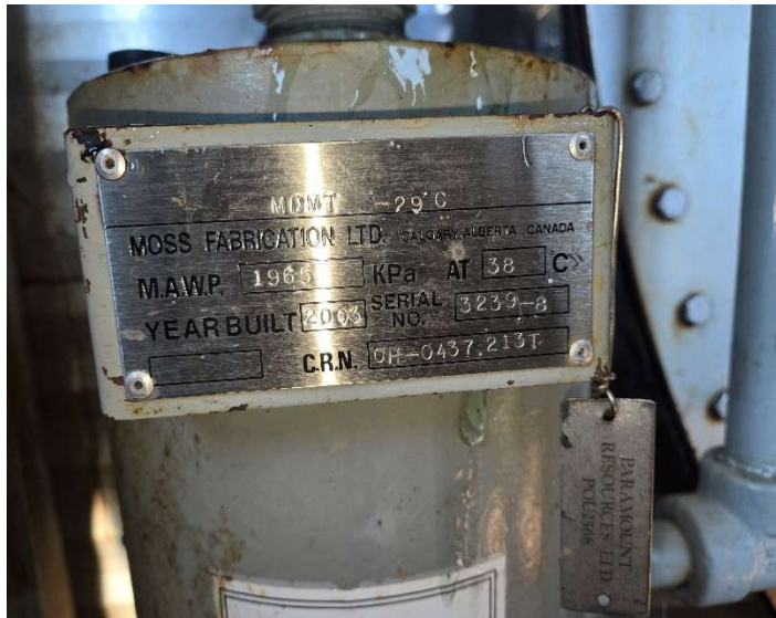
Fuel Gas Scrubber Data Plate
