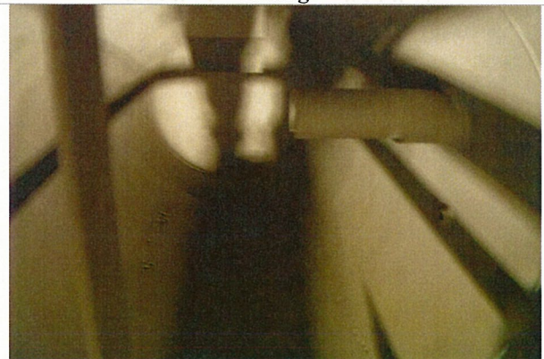
Acceptable internal Blast
