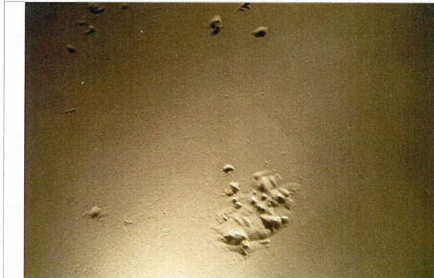
Pitting on the floor
