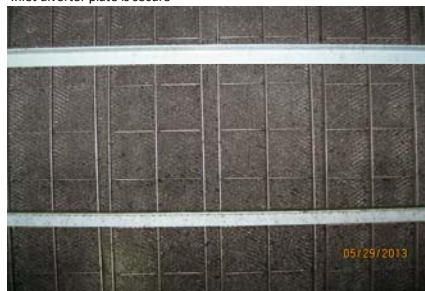
Demister material is flexible and clean of debris
