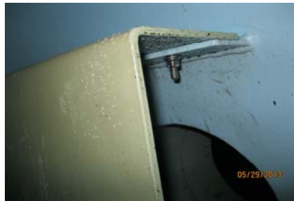
Inlet diverter plate is secure
