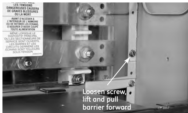
Figure 12. Horizontal bus barrier mounting slot and screw
