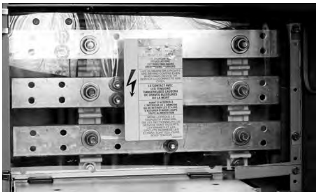
Figure 2. Horizontal bus with Lexan barrier
