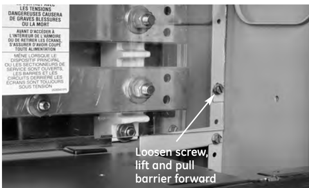
Figure 3. Horizontal bus barrier mounting slot and screw
