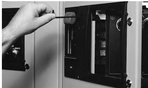
Figure 28. Concealed screw used to defeat the door interlock.
