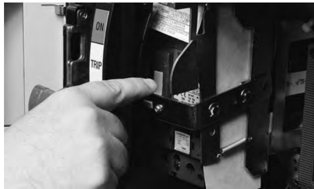
Figure 27. Door-interlock feature that prevents access to the disconnect when the power is ON.
