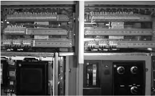
Figure 20. Typical Type C terminal boards in multiple sections
