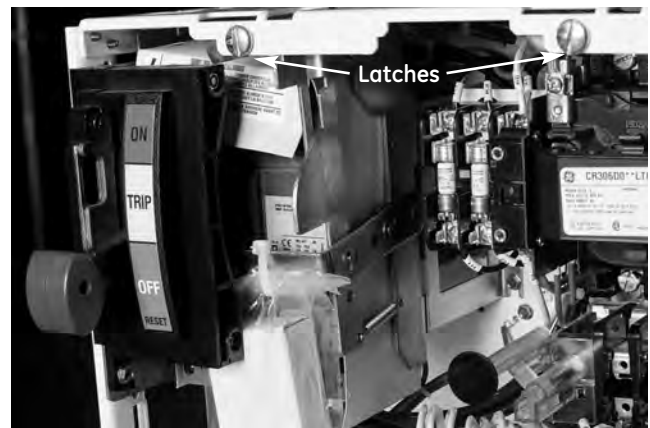
Figure 25. Unit disconnect in the OFF position. Two quarter-turn door latches are located at the top.
