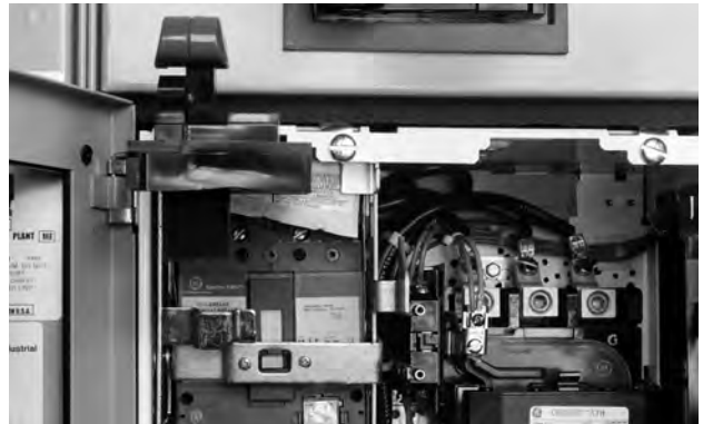
Figure 32. Rotating the operating handle to access the breaker.
