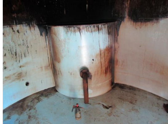
HEATER SECTION INTERNALLY
