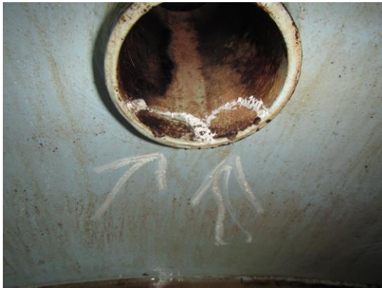
NOZZLE COATING FAILURE
