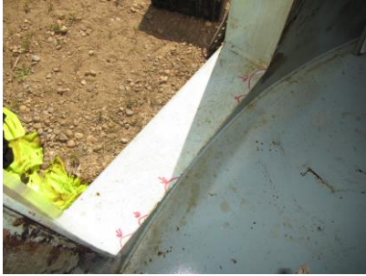
MANWAY COATING FAILURES
