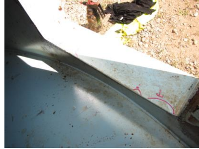
MANWAY COATING FAILURES
