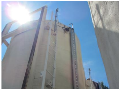
LADDER AND GAUGEBOARD
