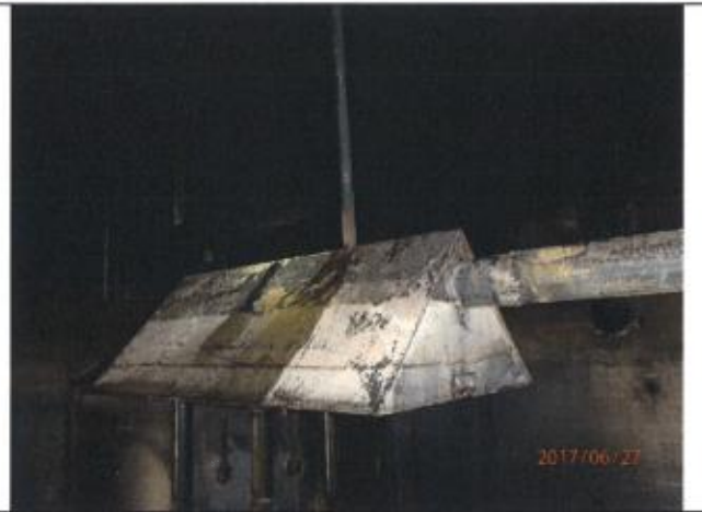
Deflector Box Overview
